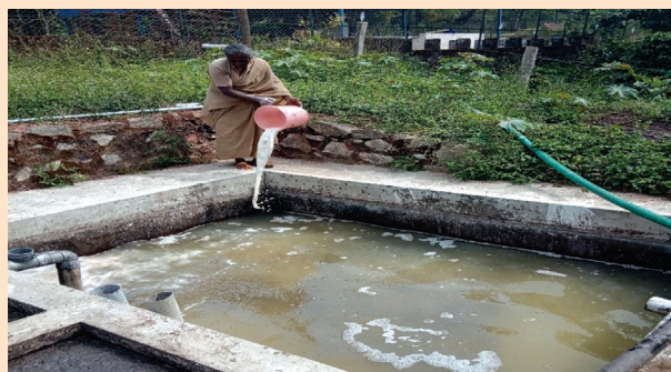
Addition of spray lime in liquid form into the equalization/neutralization tank for effective neutralization
